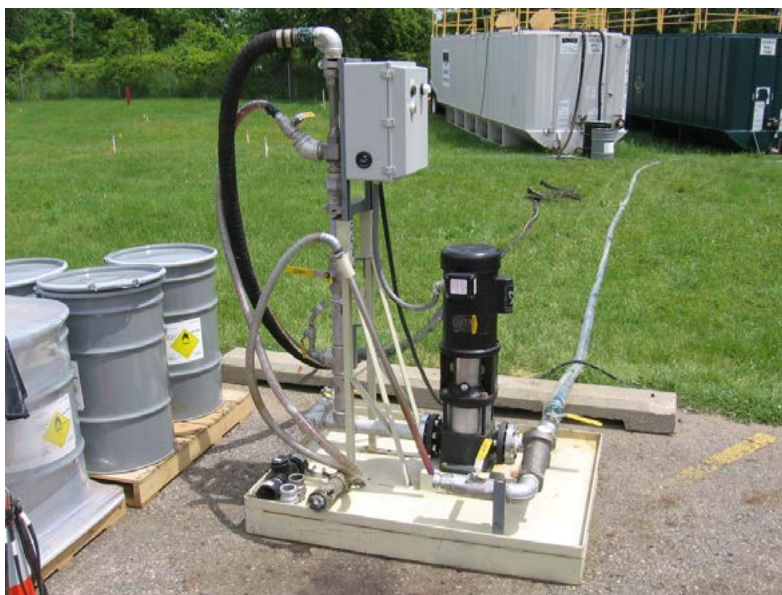
A jet pump eductor is used to mix granular potassium permanganate (drummed in foreground) with water (tanks in background). Permanganate is a common oxidant used for subsurface destruction of many persistent organic contaminants.
