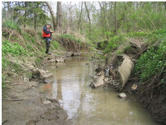
We help clients create and implement workable strategies to address water body impacts
